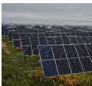
Ground-mounted solar plants
