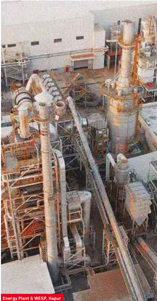
Energy Plant & WESP, Hapur
