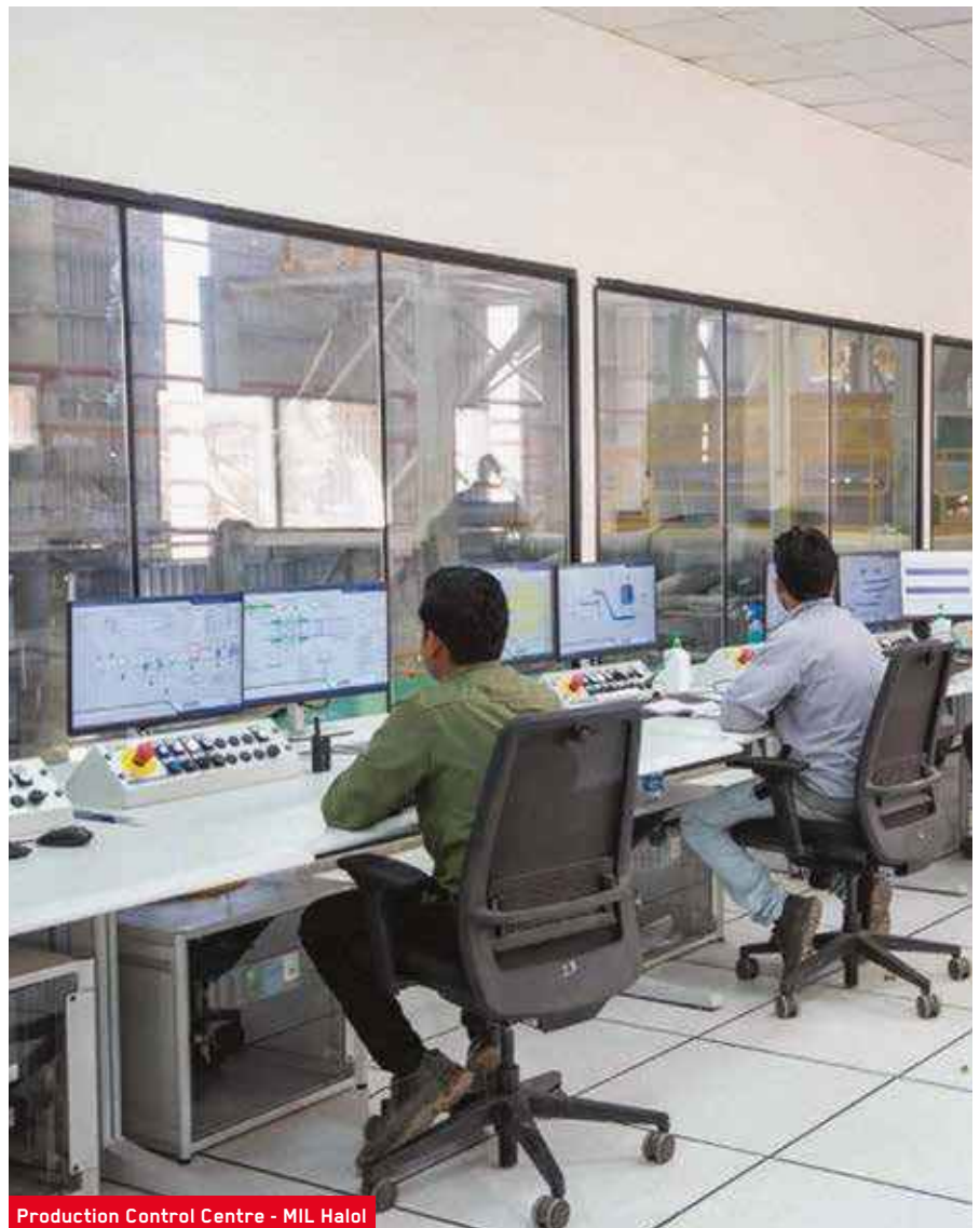
Production Control Centre - MIL Halol
