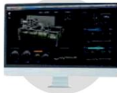
Building Automation System
