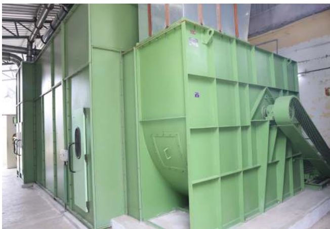
A view of new "VXL Systems" Ultra high efficiency centrifugal fan installed in our Unit at Rajapalayam.
